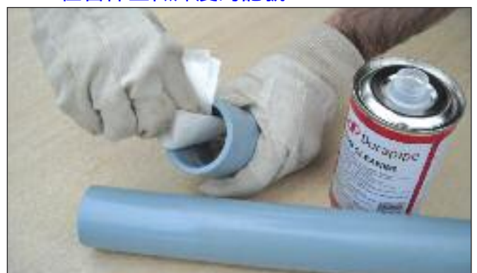
7. Clean pipe and fitting with eco cleaner. 用清潔劑清潔管件及配件
